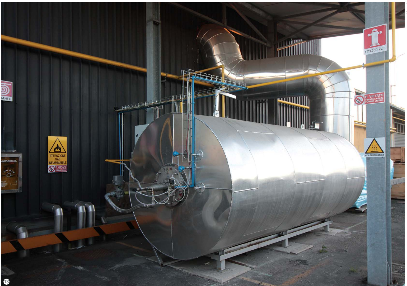
Figure 13: The energy recovery thermal afterburner.
